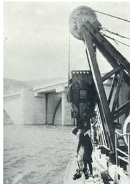
Auxiliary spillways area. 40 tons intake stop longs suspended at the service pontoon.
