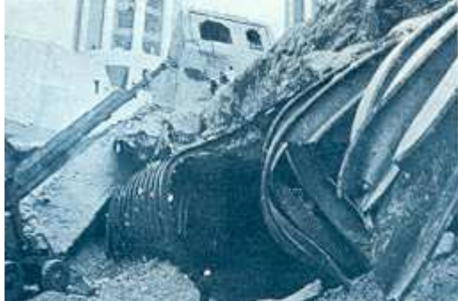
Tunnel 2. The collapsed section during removal of damaged ribs. (Courtesy of Water Power and Construction -June-July 1975)
