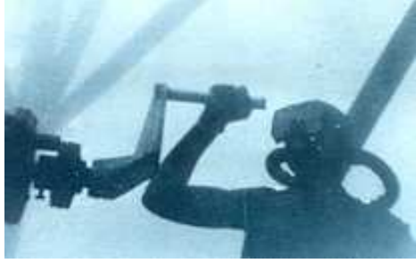
Intake tunnel 2. Hand operation of the hemispherical bulkhead's hoists
