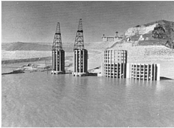
Right bank intake area. From left to right: tunnels 1,2,3,4. Note on the intake of tunnels 1 and 2 the temporary framework towers to operate the hemispherical bulkheads.
