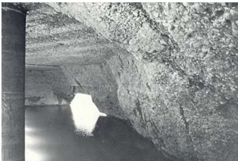
Stilling basins. Tunnels 3 and 4. eroded cavern below the middle wall.
