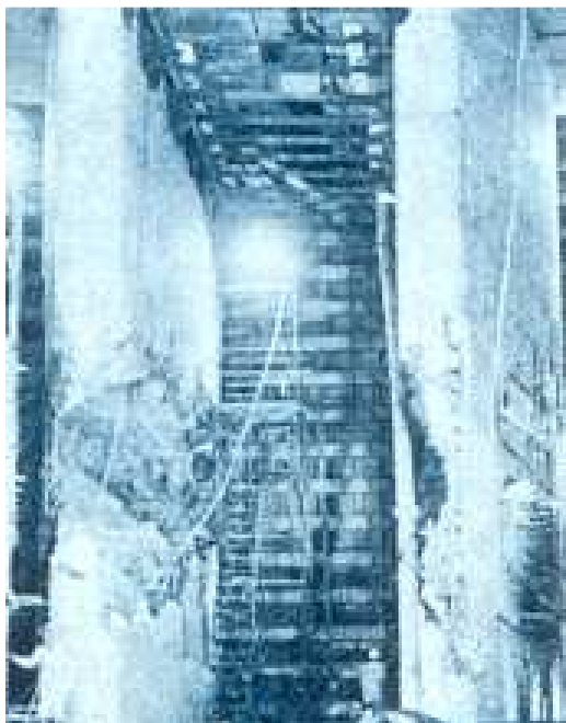
Tunnel 2. The eroded intake piers and the intake gates. (Courtesy of Water Power and Dam Construction – June-July 1975)
