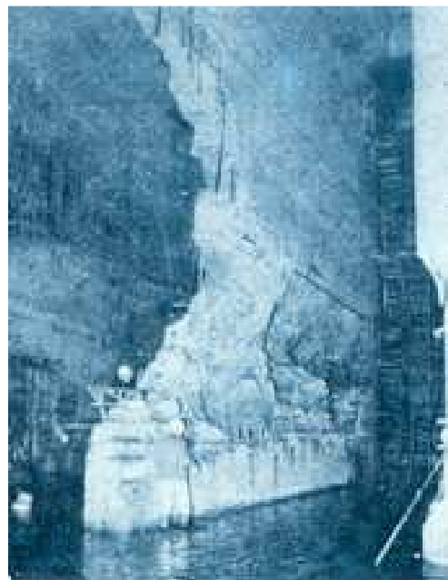
Tunnel 1. Intake piers after dewatering. (Courtesy of Water Power and Dam Construction – June-July 1975)
