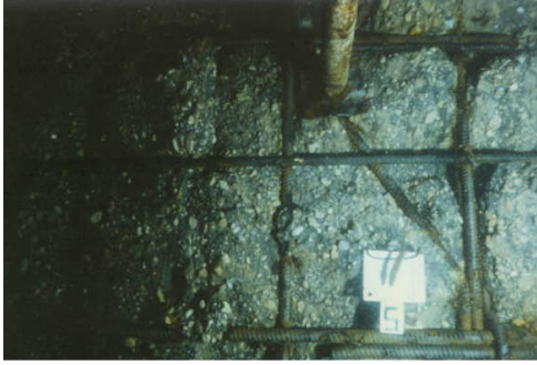
Underwater exposed reinforcement after grit blasting
